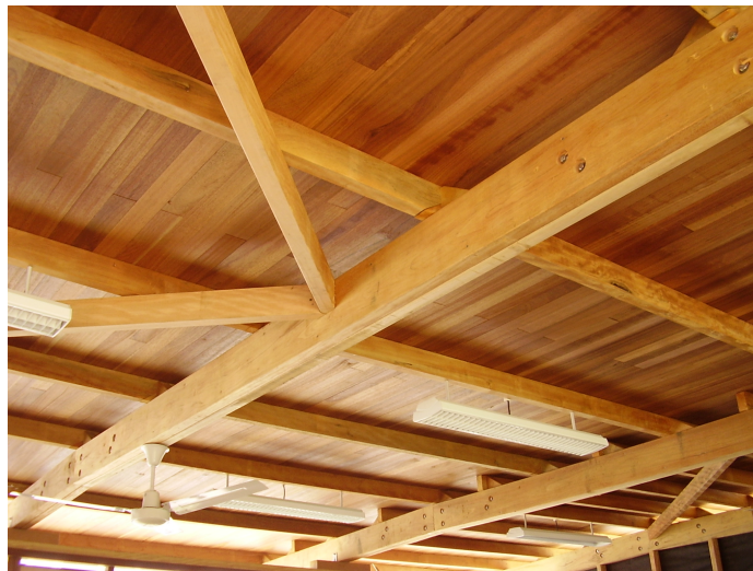
Basralocus sheathing on a ceiling frame in Mandioqueira, Gontran Damas secondary school, Cayenne (French Guiana).
